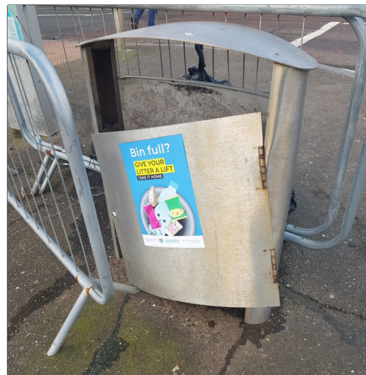
6. Pier Head: near the John Muir Way Start/End Point. Broken hinges and missing base of bin.
